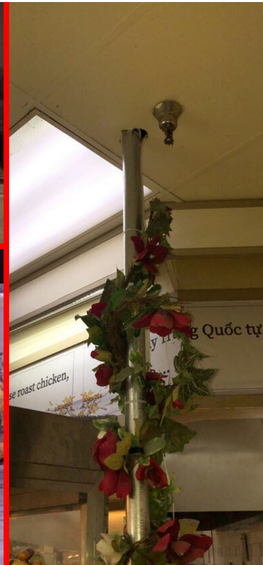
Penetration into ceiling
