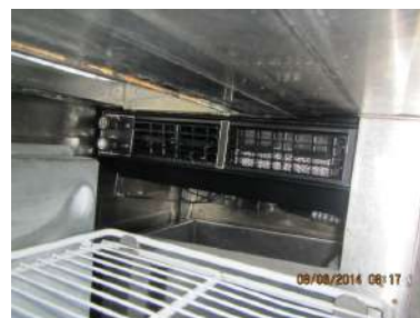
Cold plate refrigeration
