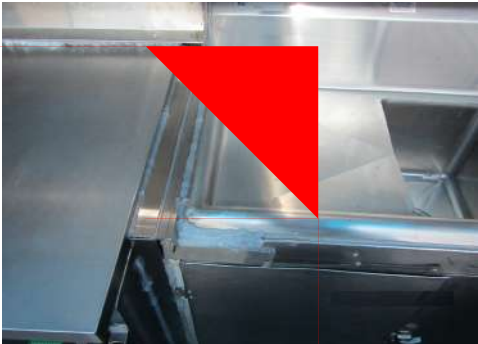
Sloppy, uneven caulking. Not smooth or easily cleanable.
