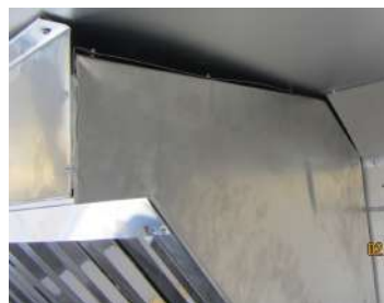
Hood not properly installed
