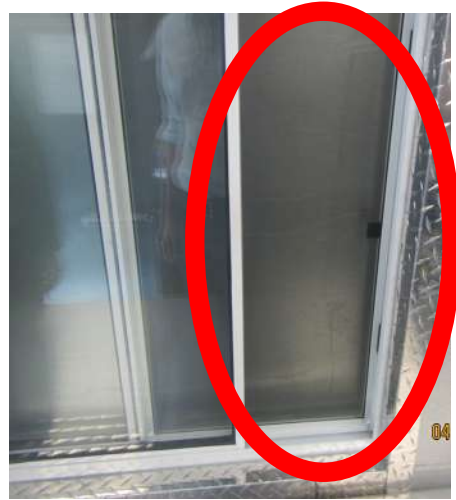
Opening is too large (See chapter 5)
