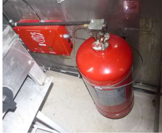
Approved automatic fire suppression system
