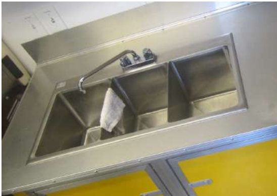
No drain boards
