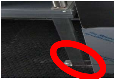
Equipment properly sealed to the floor
