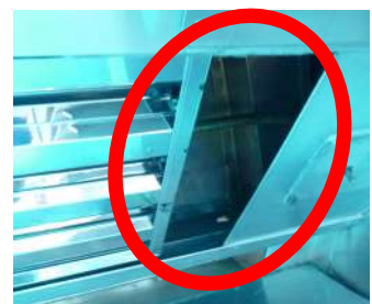
Gaps in filters
