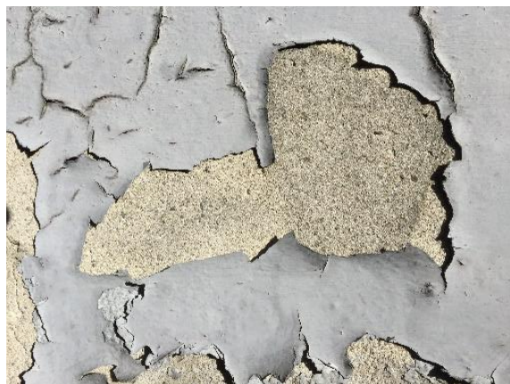
Figure 2. Peeling Lead Paint
