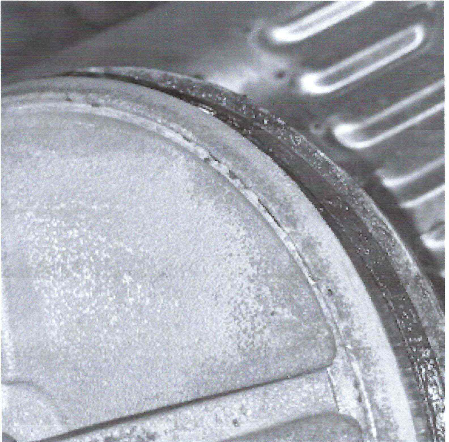
worn / flattened seal
